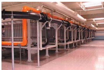
Courtesy Photo: Siemens
