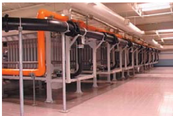
Courtesy Photo: Siemens
